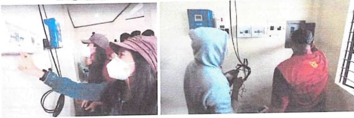
Installed Solar Controls, Breakers and Switch
